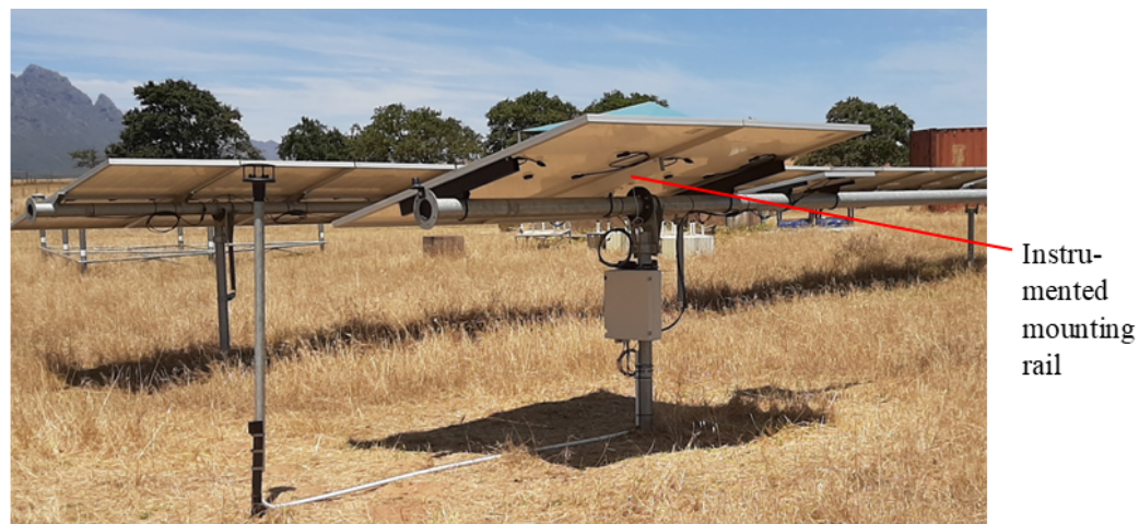
Figure 2. Experimental setup added to the existing SAT PV array
